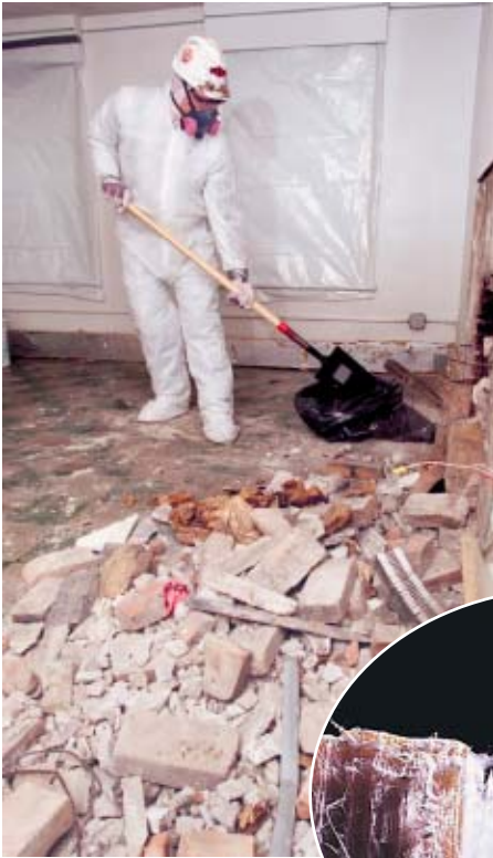
Figure 10 ▶ Asbestos (right) forms in long, thin fibers. The worker above is removing debris from a structure that was built with asbestos.
